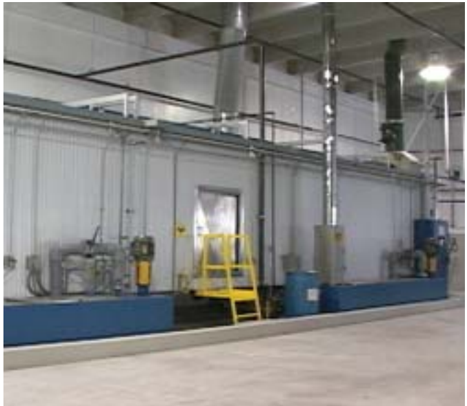
The three-stage washer provides the critical preparation needed for outdoor performance of powder on aluminum. (Photos courtesy of National Partitions)
