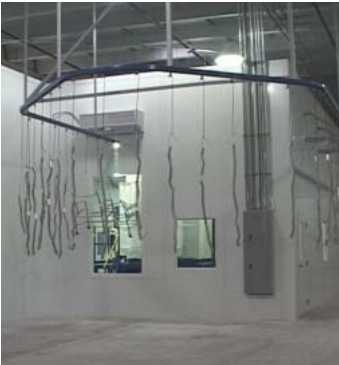
The environmental room controls the heat and humidity for precise application control.
