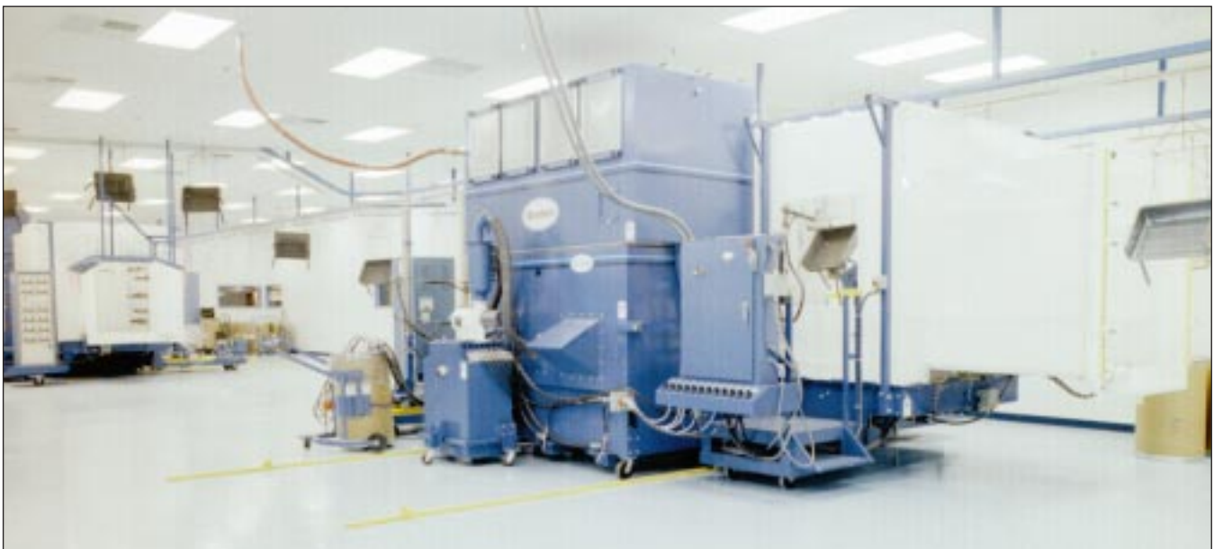
Two powder booths can be rolled on and off the same line for fast color changes. (Photo courtesy of Nordson)
