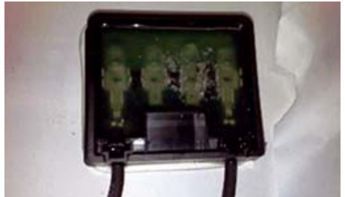
Soldered connective sockets
